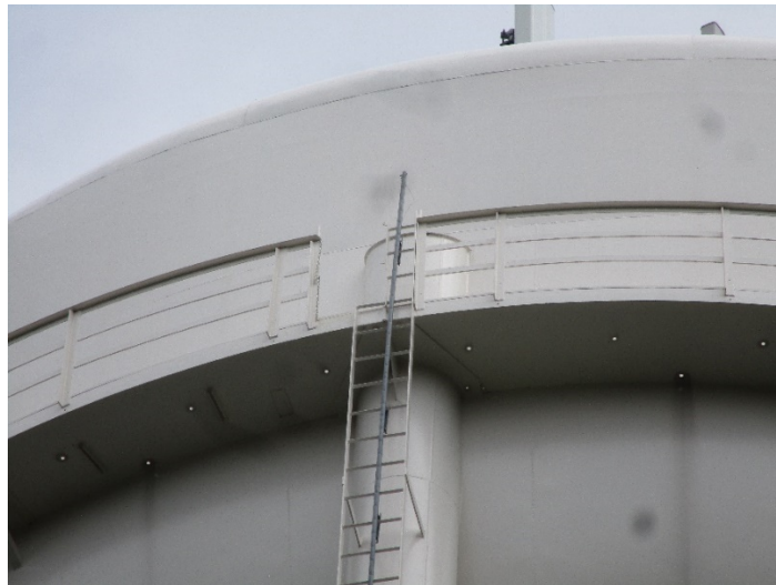
Muir's Chapel Tank shown (similar condition at Gate City Boulevard Tank)
