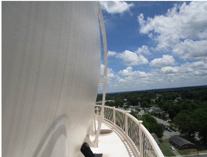
Gorrell Street Tank shown (similar condition at Lees Chapel Road Tank and Gate City Boulevard Tank)
